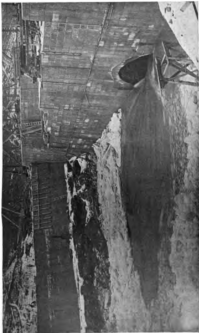
PLATE 43—View of Upstream Face of Olive Bridge Dam during Construction. Spring Freshet Passing through Culvert in Dam.
